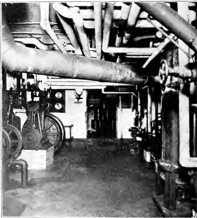
FIG. 7. VIEW OF ENGINE ROOM, JACQUES KAHN, INC., SHOWING FEEDWATER PUMPS AND FEEDWATER HEATER
